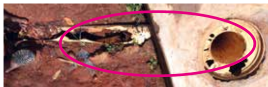
Figure 3. Broken pipe, not submerged as required by terms of reference
